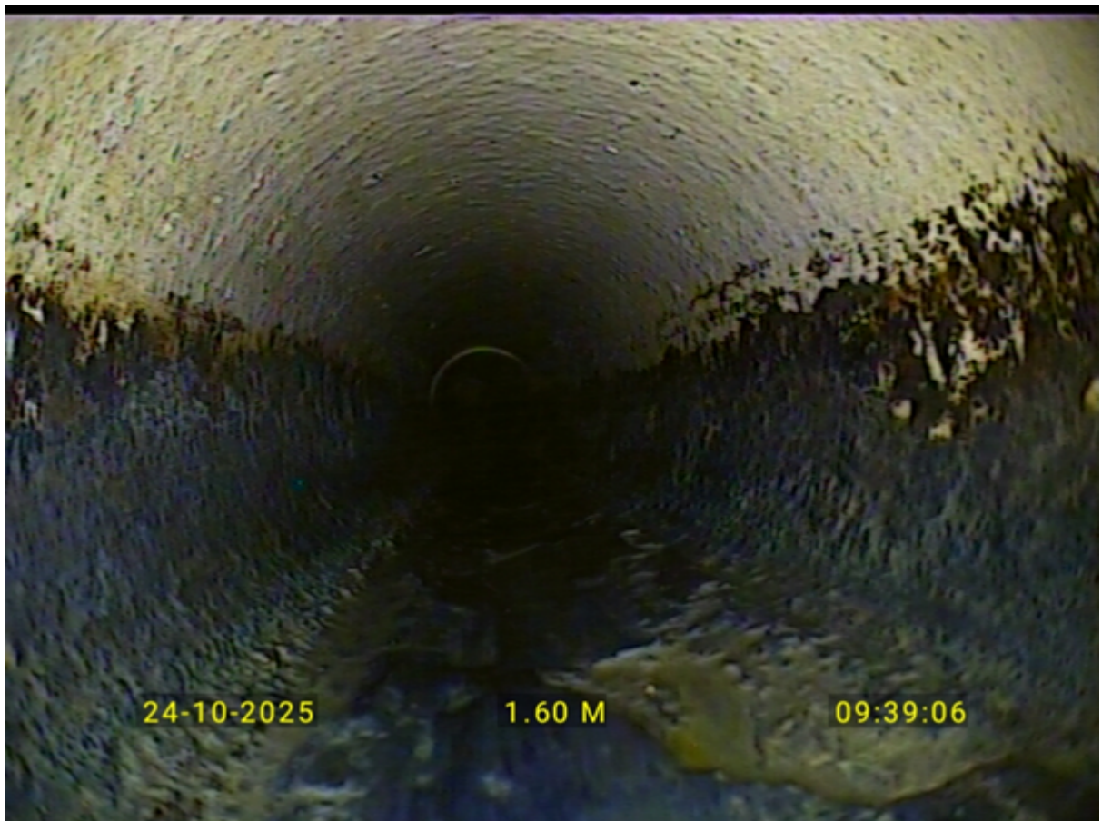
Heavy scale on urinal pipe run
