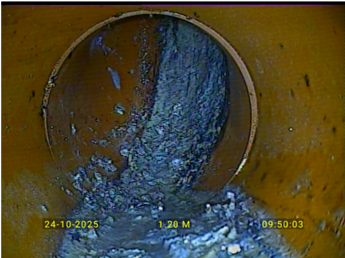
Scale in urinal pipe
