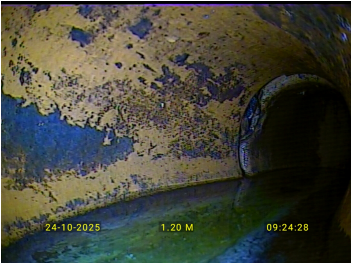
There were some misaligned joints and standing water in the disabled pipe run, which may point to insufficient fall.
