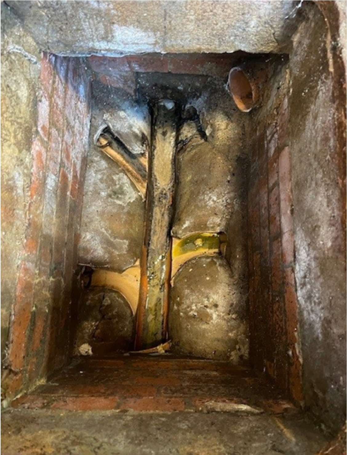
Blockage clear and showing heavy scale
