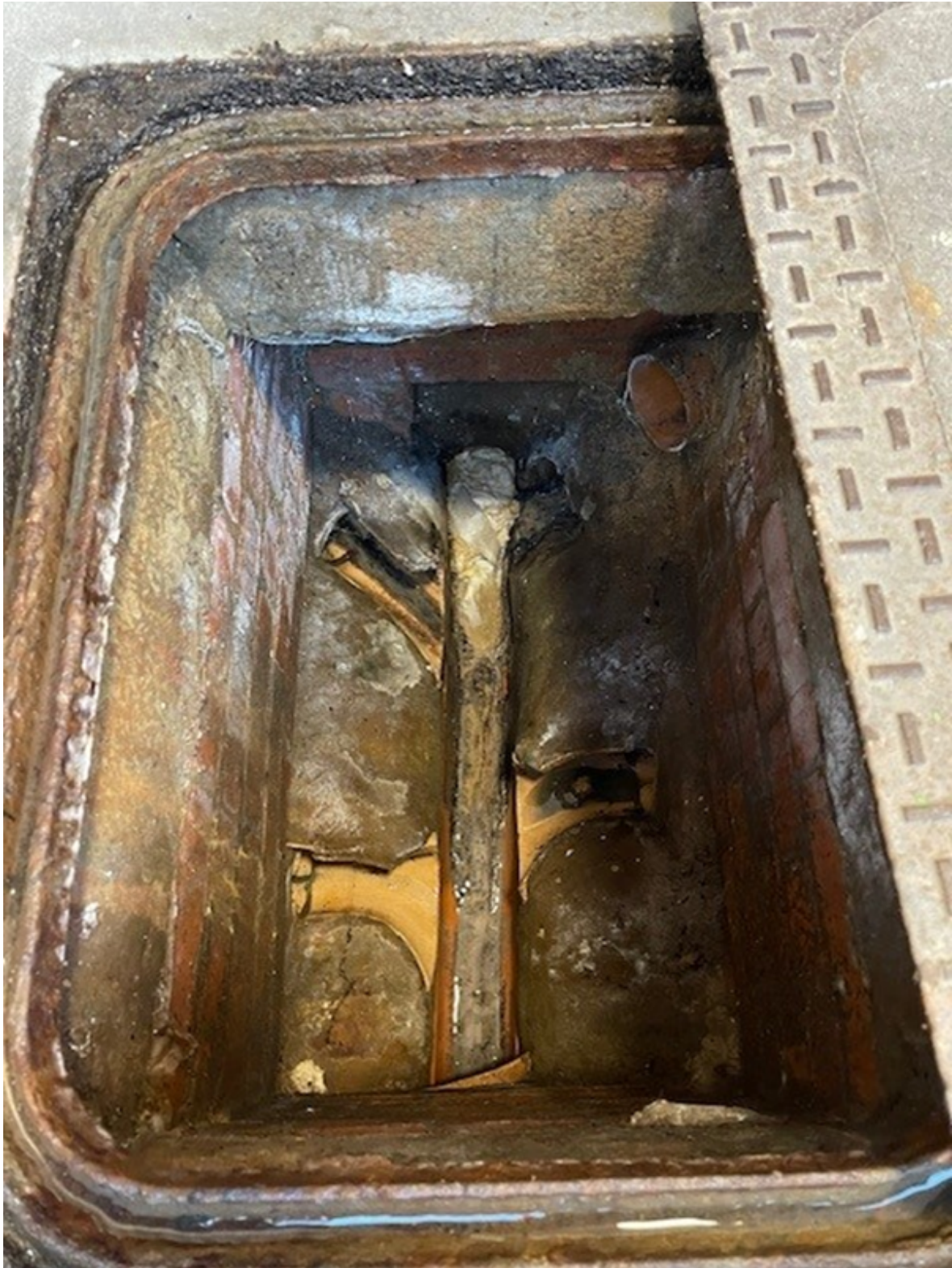
Inspection Chamber with blockages
