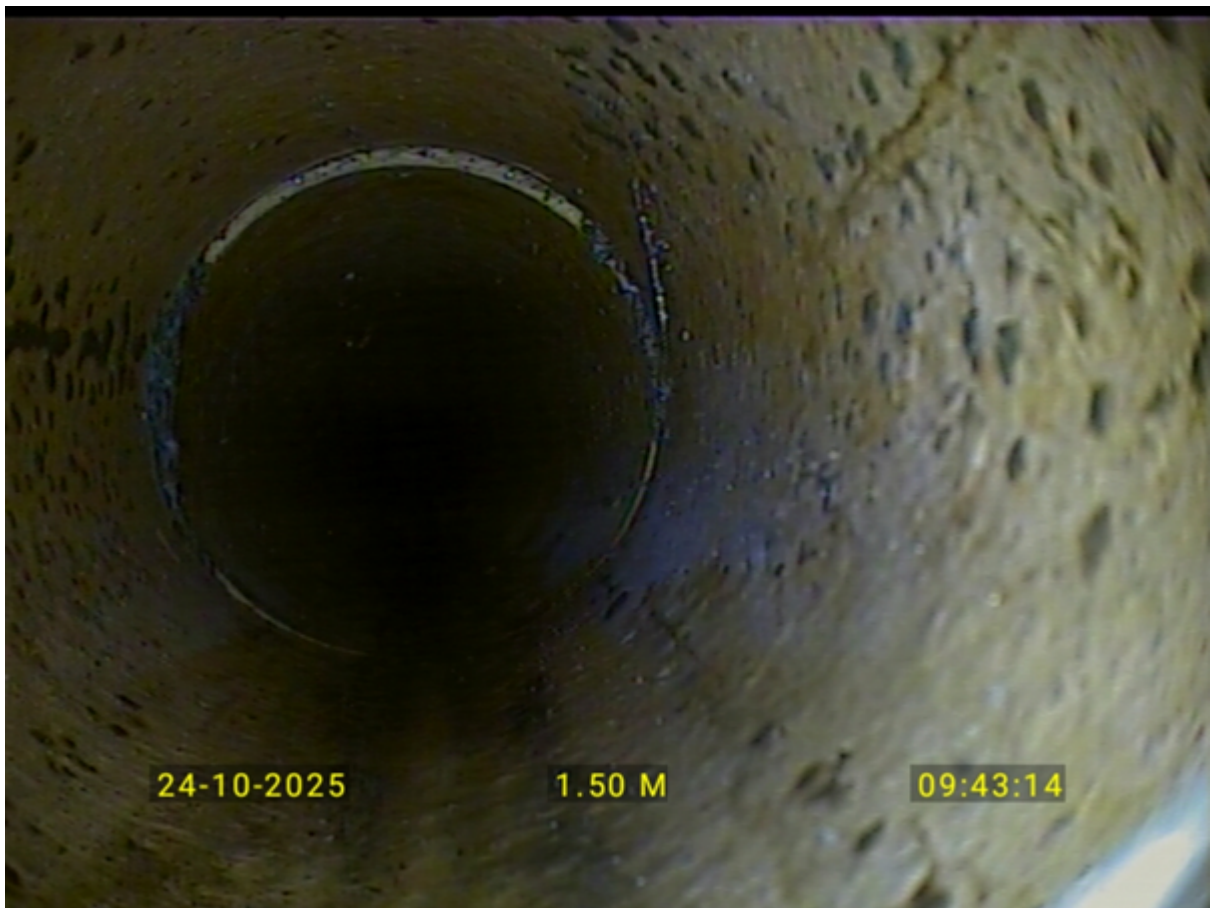
Minor misalignment on gents basin run
